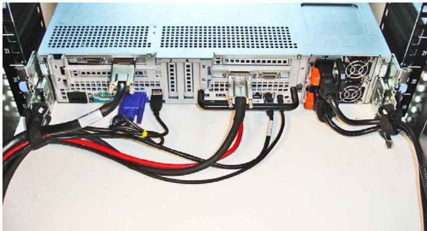
Figure 6: Cable Routing Without a CMA
